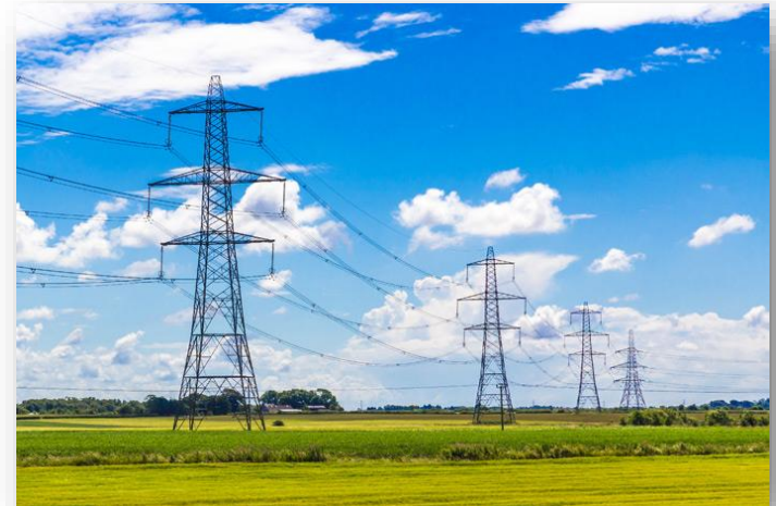
Pylons carry overhead power cables
