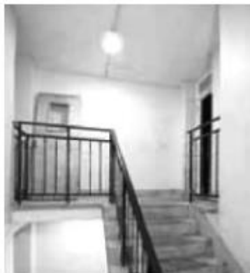
photo of stairwell with LED fitting
